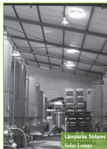
Paneles Solares Solar Panels
